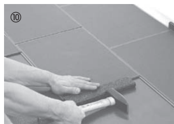
Then you interlock the board with the board to its left at the short side, using hammer and tapping block or, in hard-to-reach areas, the pull tool.
