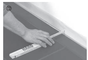
Cut to size and fit the last row. Leave a gap of 10 to 15 mm between the boards and the wall.
