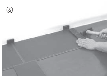
Join the boards of the first row at the short sides using hammer and tapping block. It is important to ensure that the first row is straight and exactly parallel to the wall.
