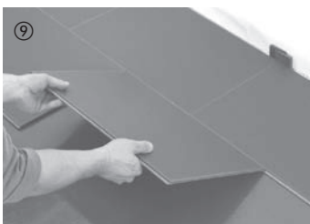
The remaining rows should be installed board by board. First, the board is angled into the previous row along the long side by applying a small amount of force.
